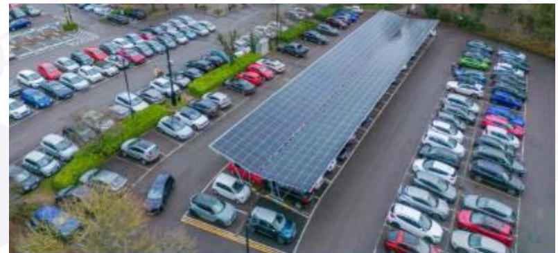
Aerial view of the solar carports at Kingfisher Leisure Centre in Sudbury. Babergh District Council/ Simon Watson Photography (Image: Babergh District Council/ Simon Watson Photography)
