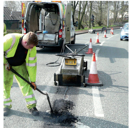
Failed Joint Heater 2 x 0.5 (APSE May/June 2011)
