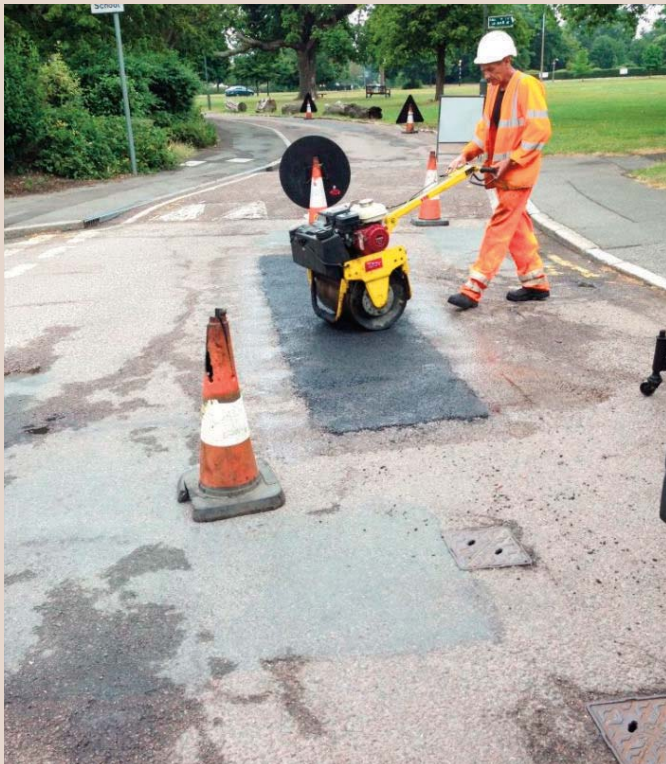
Thermal repair's being carried out in Croydon, 2 year old Nu-phalt repairs in the foreground
