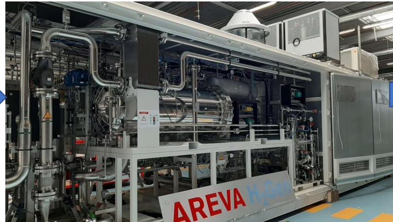
500-kW Areva electrolyser
