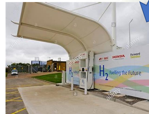
Bus fuelling depot, Belfast Translink
