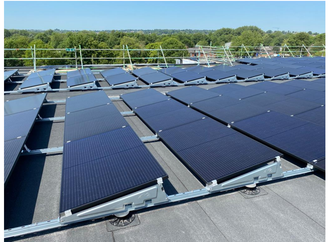
150kWp at WCC New Leisure Centre
