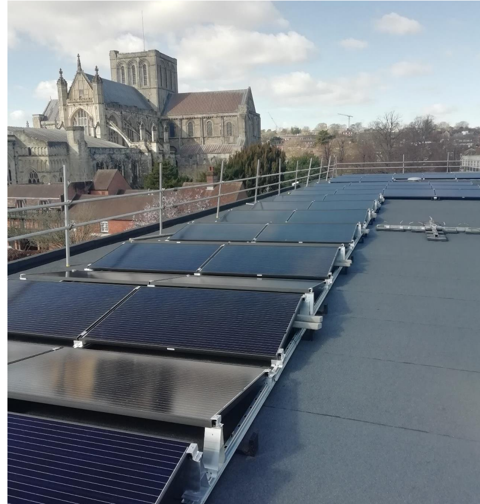
50kWp at Civic Offices
