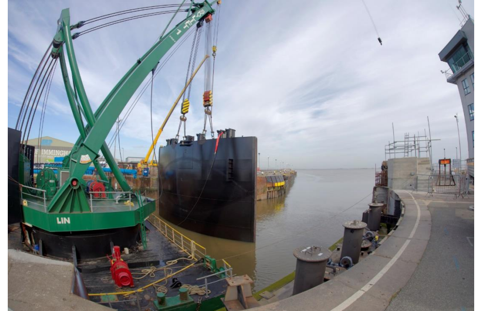
Port of Immingham £7.4m scheme to improve flood defences after tidal surge in 2013.
