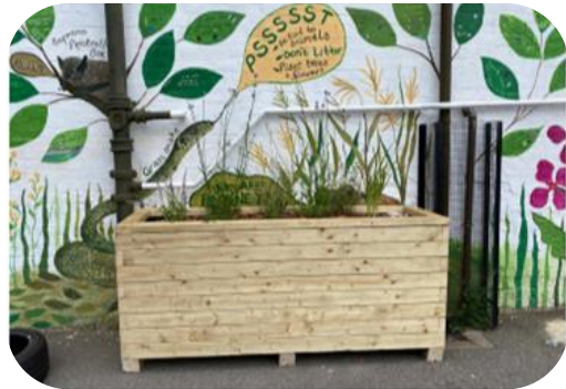
571 SuDS Rain planters at the end of downpipes across 71 schools
