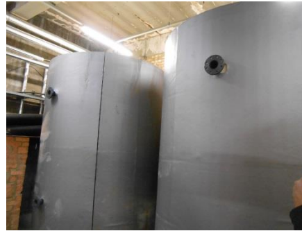
Two 10,000 litre buffer tanks £19,000
