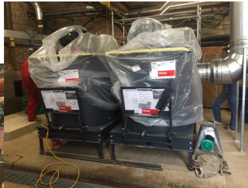
Gas boilers and pipework £190,000
