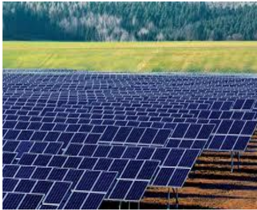
Electricity Generation facility
