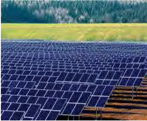
Electricity Generation facility
