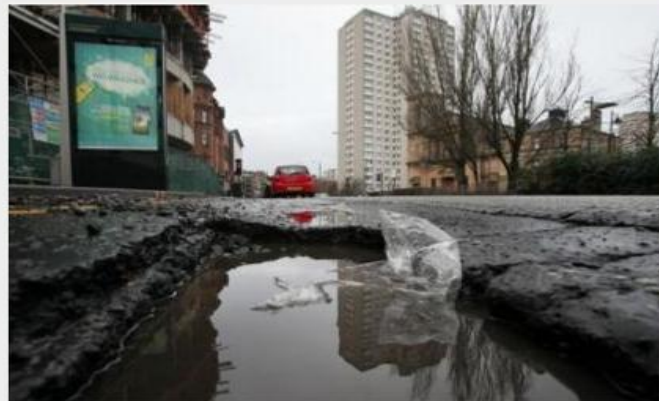
Thousands of potholes have been repaired, but not this one in Cowcaddens Road
