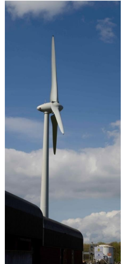
ASC Renewables project at Newton Marsh sewage works
