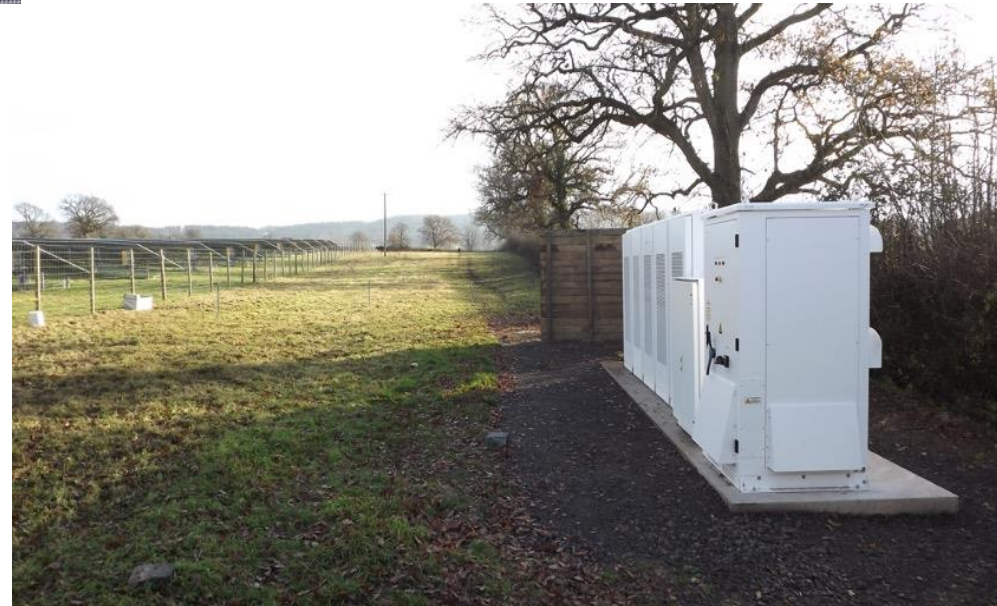
CES's Battery Energy Storage project, utilising Tesla's Powerpack solution, alongside existing Solar PV site.
