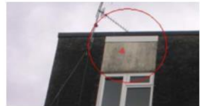
Figure 6: mould on saturated render panels
