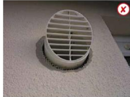
Figure 34: Unsealed extract fan in a bungalow
