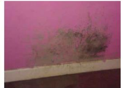
Figure 53: Damp behind a bed, removed for inspection
