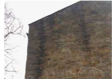
Figure 14: Staining from roof water run off
