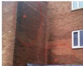
Figure 5: mould on saturated brickwork
