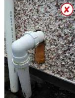
Figure 35: Unsealed pipe penetration
