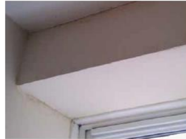
Figure 50: Damp in the kitchen
