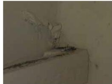
Figure 52: Damp in the wardrobe
