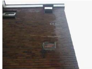
Figure 13: Wall staining from water blown off the roof
