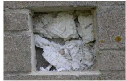
Figure 4: Example of saturated insulation
