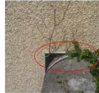
Figure 48: Plant growth allowed by poor detailing
