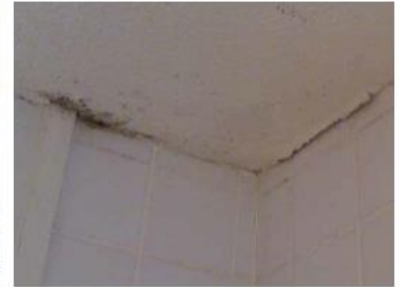
Figure 51: Damp in the bathroom
