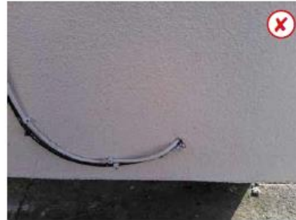
Figure 36: Unsealed wire penetration
