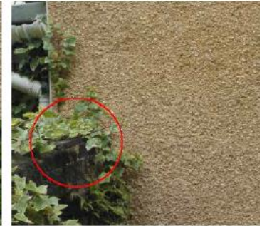
Figure 49: Close proximity of plant requiring pruning
