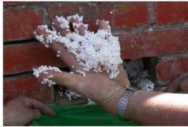
Figure 3: Example of saturated insulation
