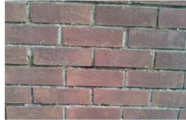
Figure 11: Erosion of mortar by weather
