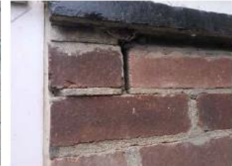
Figure 12: Cracked and missing
