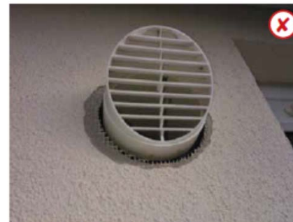
Figure 34: Unsealed extract fan in a bungalow
