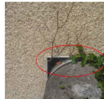
Figure 48: Plant growth allowed by poor detailing
