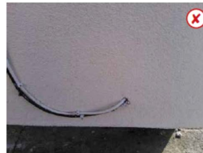
Figure 36: Unsealed wire penetration
