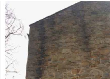
Figure 14: Staining from roof water run off
