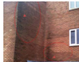
Figure 5: mould on saturated brickwork
