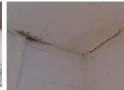
Figure 51: Damp in the bathroom
