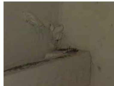
Figure 52: Damp in the wardrobe
