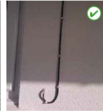
Figure 39 - cable clipped (good practice)
