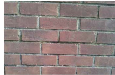
Figure 11: Erosion of mortar by weather
