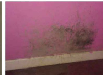
Figure 53: Damp behind a bed, removed for inspection
