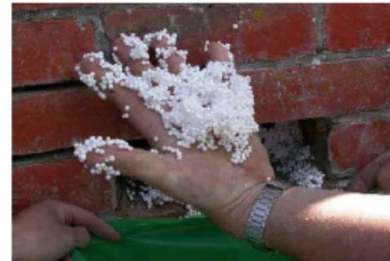
Figure 3: Example of saturated insulation
