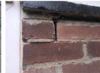
Figure 12: Cracked and missing
