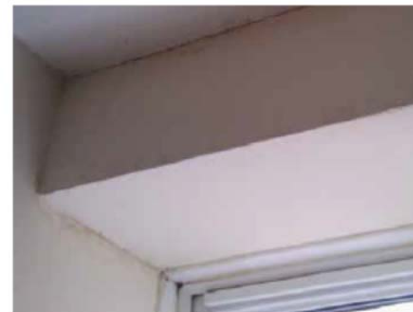
Figure 50: Damp in the kitchen
