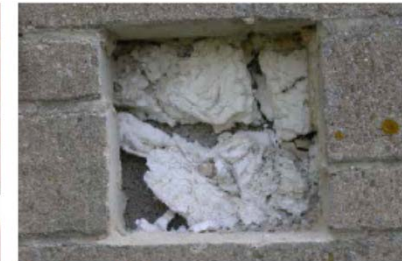
Figure 4: Example of saturated insulation
