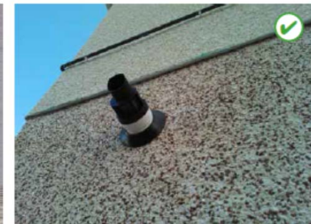
Figure 37: sealed penetration (good practice)
