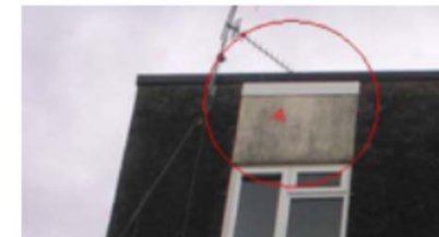
Figure 6: mould on saturated render panels
