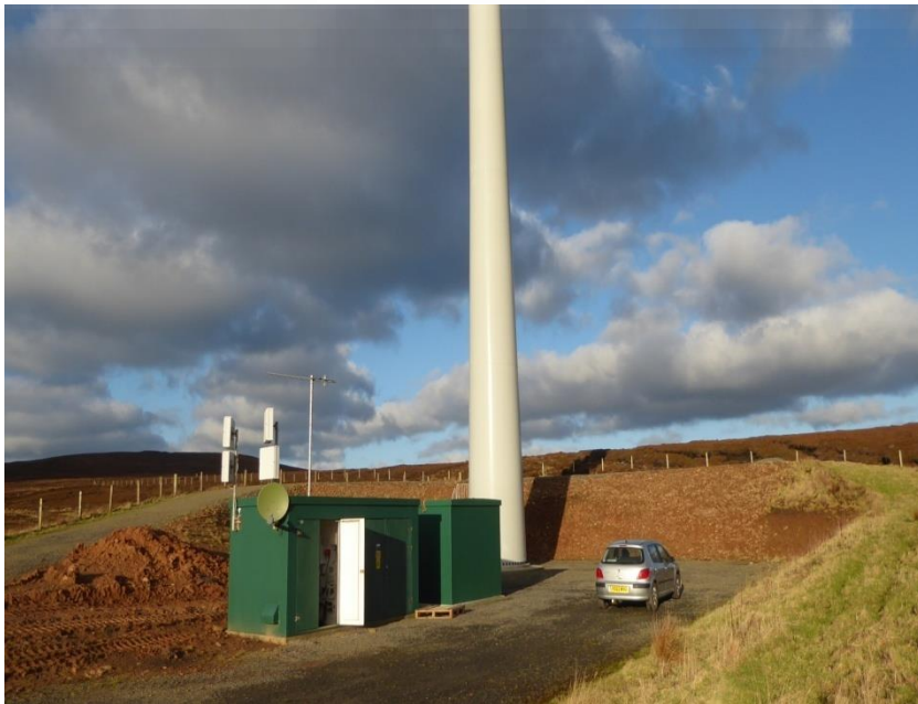
ERE turbine and switchgear
