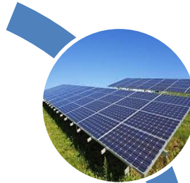
Solar PV farm
