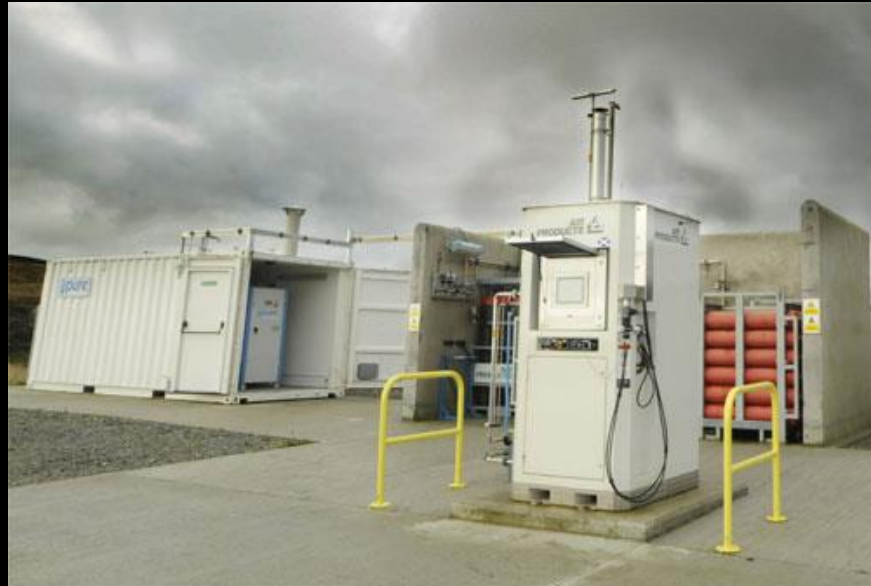
CnES Outer Hebrides Local Energy Hub facility at Creed
