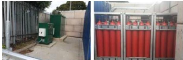
Electrical kiosk and transformer
