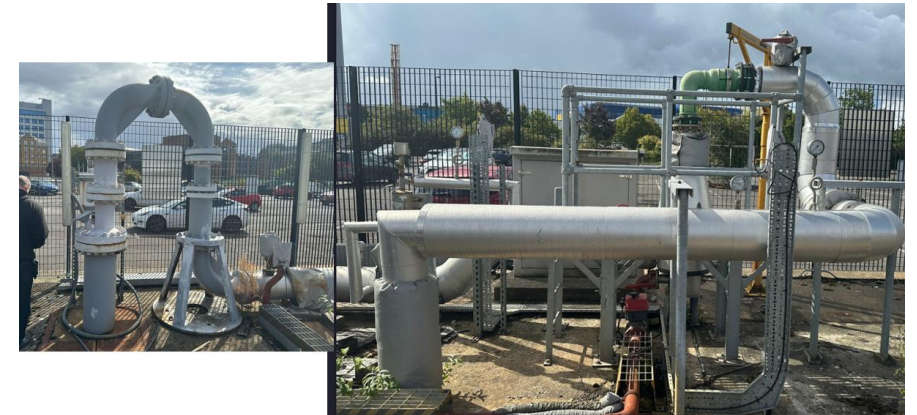
Left: well head, right: cyclone and buried pipework to Energy Centre
