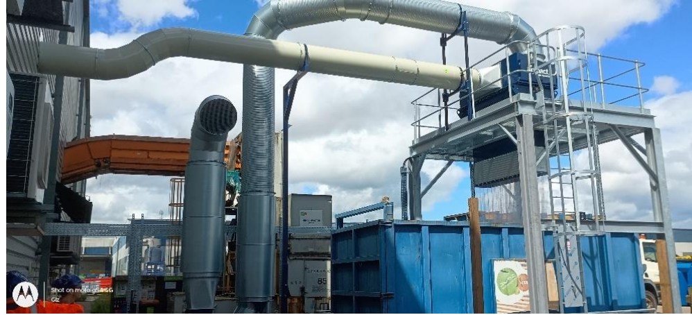
Vacuum extraction system – Suez, Avonmouth (S. Gloucestershire)
