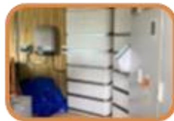
Osney Lock Hydro battery
