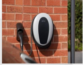
EV Charging points
