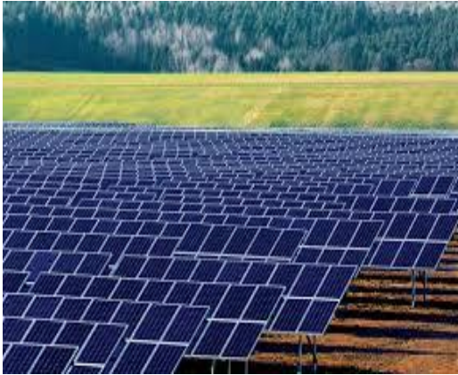
Electricity Generation facility
