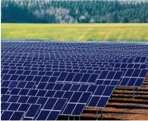
Electricity Generation facility
