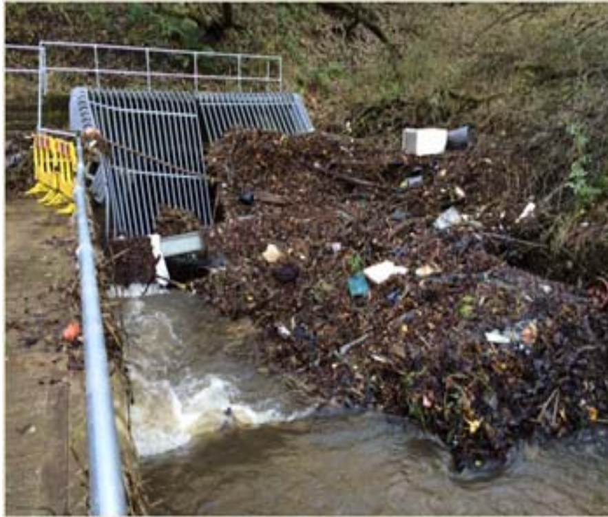
Hebble Brook trash screen failure.
