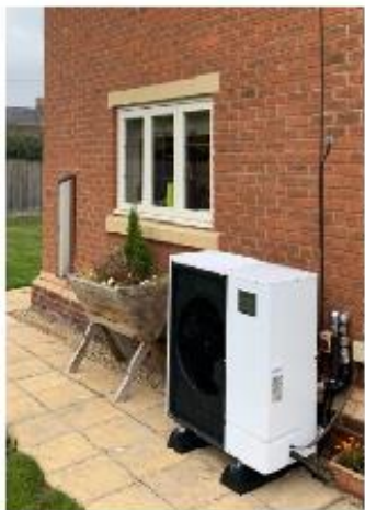
Air Source Heat Pump
