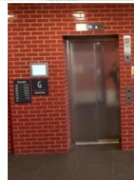
Landlord Supply to residential lift.
