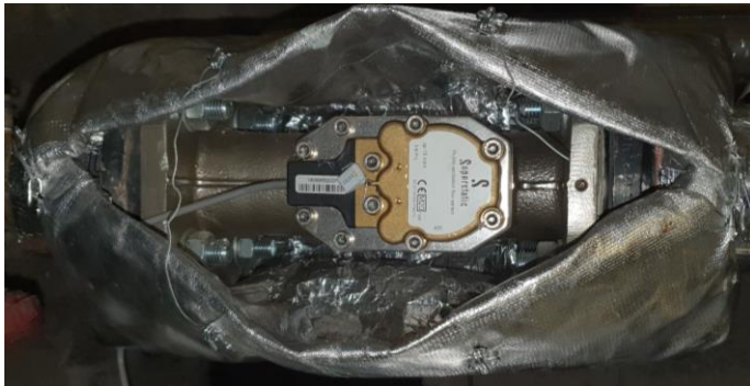
Heat Meters (and Electrical Meters)
