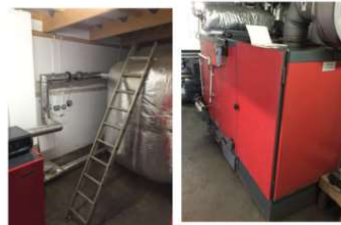
Figure 6: 92kW Binder biomass boiler and buffer tank
