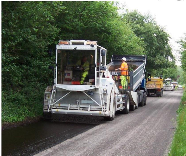
Figure 8.1 Rural Road 10 mm Racked-in with 6 mm Surface Dressing Intermediate Polymer Modified Binder
