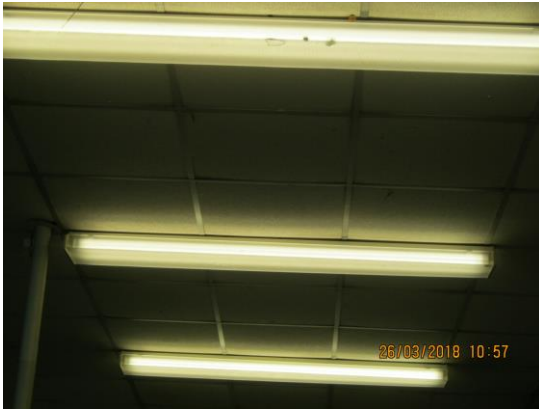
6ft T8 Lighting = High energy saving potential
