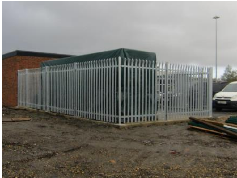
2MW Tesla Battery
