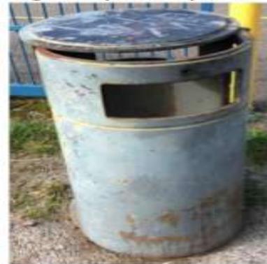
Grade D Urgent repairs required
